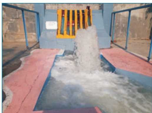
Flow conditions D/s of spillway in the scour pit
